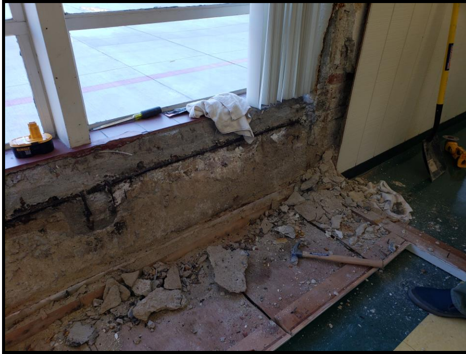
Photo #3 – Damage at bottom corner of window
