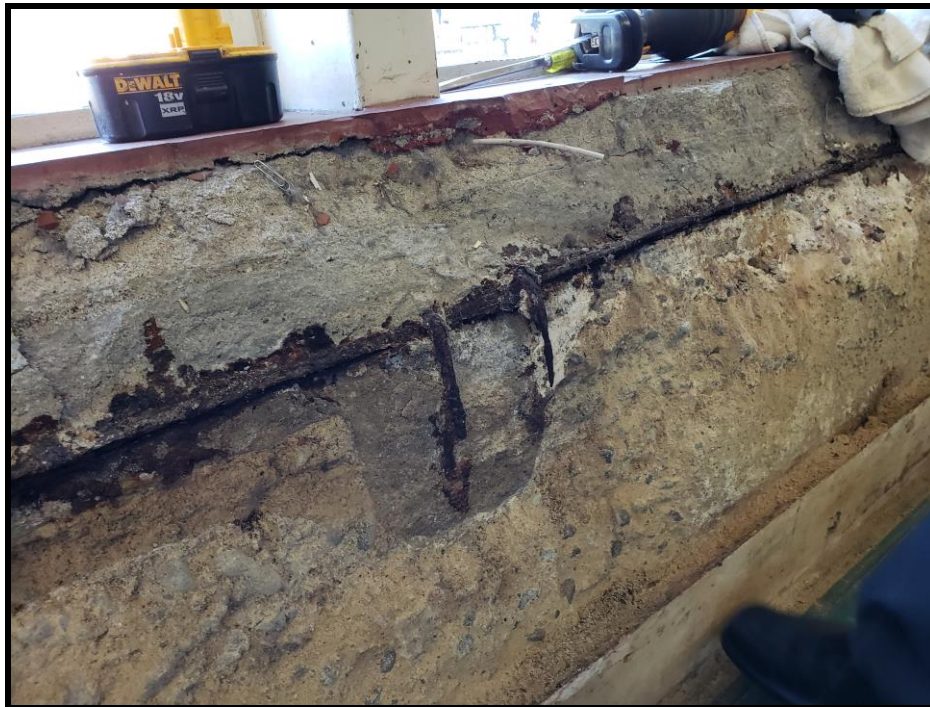
Photo #4 – Rusted rebar at window mullion
