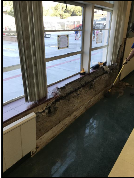
Photo #1 – Part of affected area with surface panels removed.
