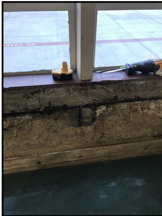
Photo #2 – Damage under window mullion with rusted rebar
